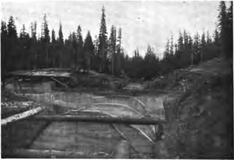
FIG. 173.—Outlet Conduit, Keechelur Dam, Washington, Showing Concrete Cut-off Collars, Corewall and Track for Backfilling on Left.
